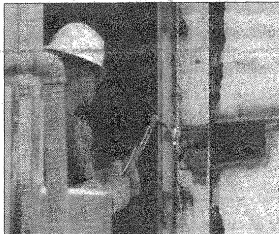
A TNT Excavating crewman uses a cutting torch to prepare one of the two silos for demolition. (Tom Compton photo)
